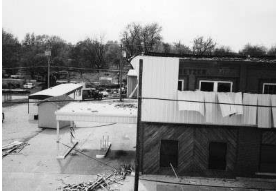
Plate 2.1 Severe wind damage to structure.
