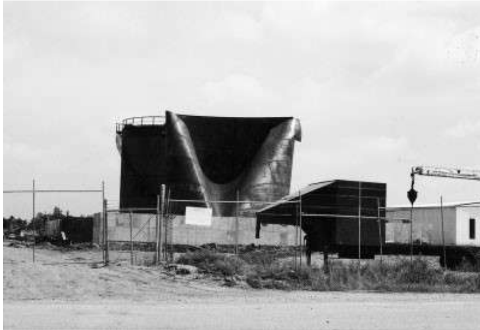
Plate 2.2 Relatively moderate wind caused collapse of tank during construction due to insufficient bracing.
