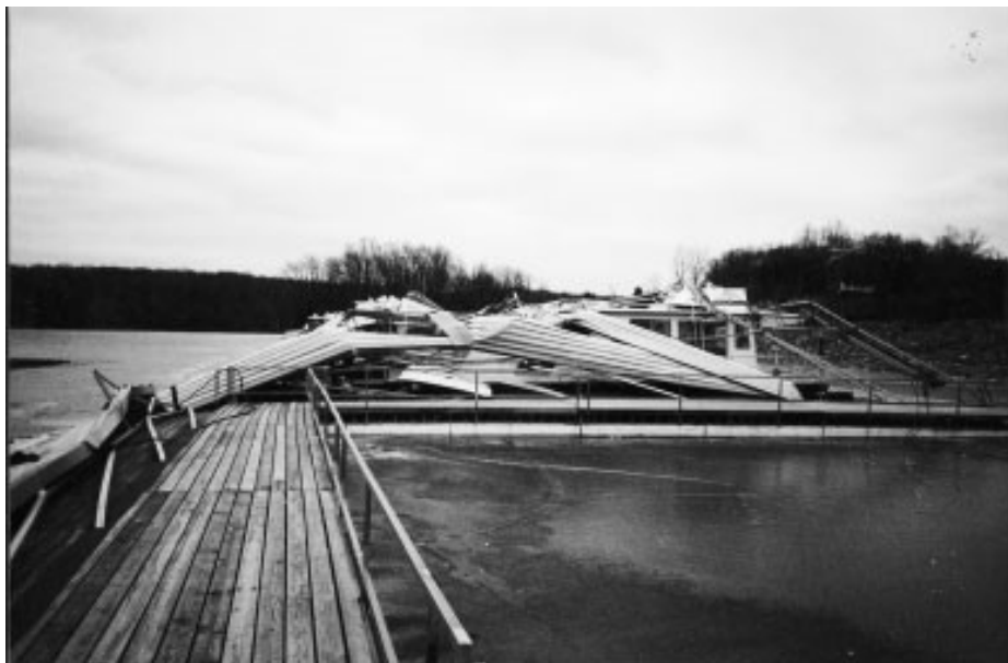
Plate 2.3 Roof over boat docks loaded with ice and snow, collapsed in moderate wind.
